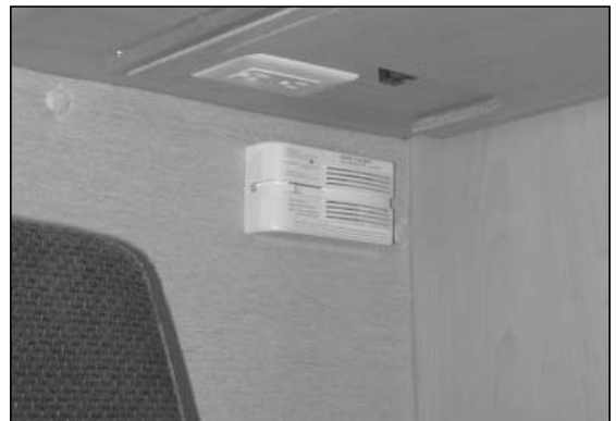
Picture F-P2: Carbon monoxide leak detector.
